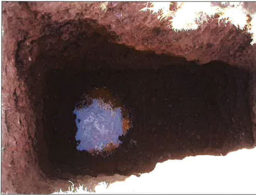
Photo 3: Ground Water Seepage in Test Pit TP5
